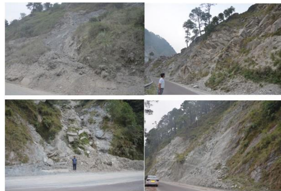
Fig. 5 Field photographs showing the various types of slope failures in the study area.
